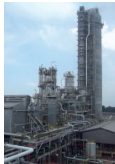
1,725 MTPD ACES21™ urea plant of PT Pupuk Kujang
