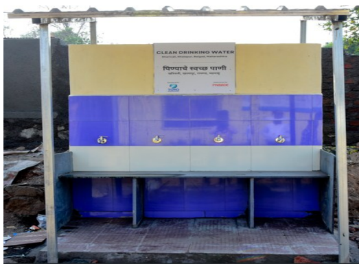
Clean drinking water system
