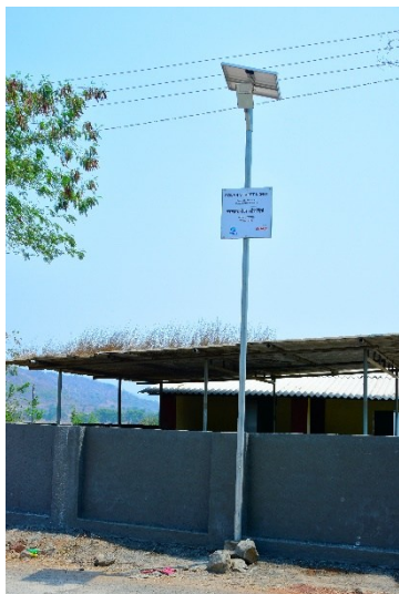
Solar street lights
